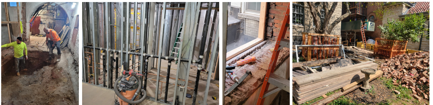
During the week the sound of the jackhammer echoes throughout the campus as workers dig out the shaft for the elevator to rise in the Parish House. Aluminum studs outline the space for new restrooms. Century-old window frames will be reclaimed. And the east garden is now a construction site that will rebloom with a ramp to the elevator.
